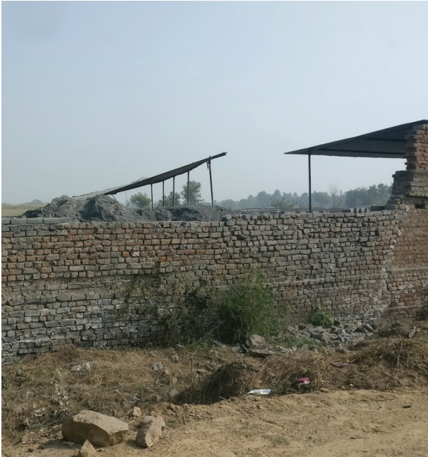
Inadequate height of a boundary wall at a unit in Gurugram
