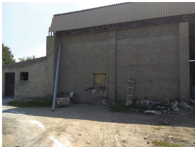
Inlet pipe at the front wall to connect to the bulkers
