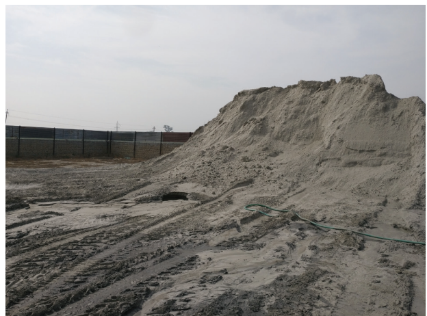
Unpaved passage for trucks to the storage area at a plant in Jhajjar
