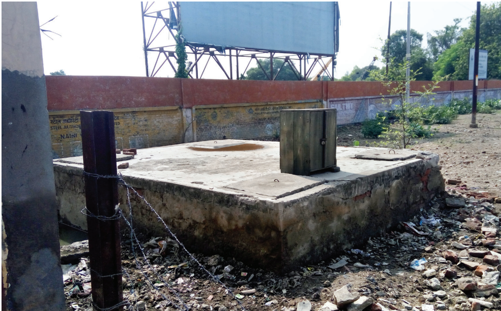
Septic tank connected to open drain
