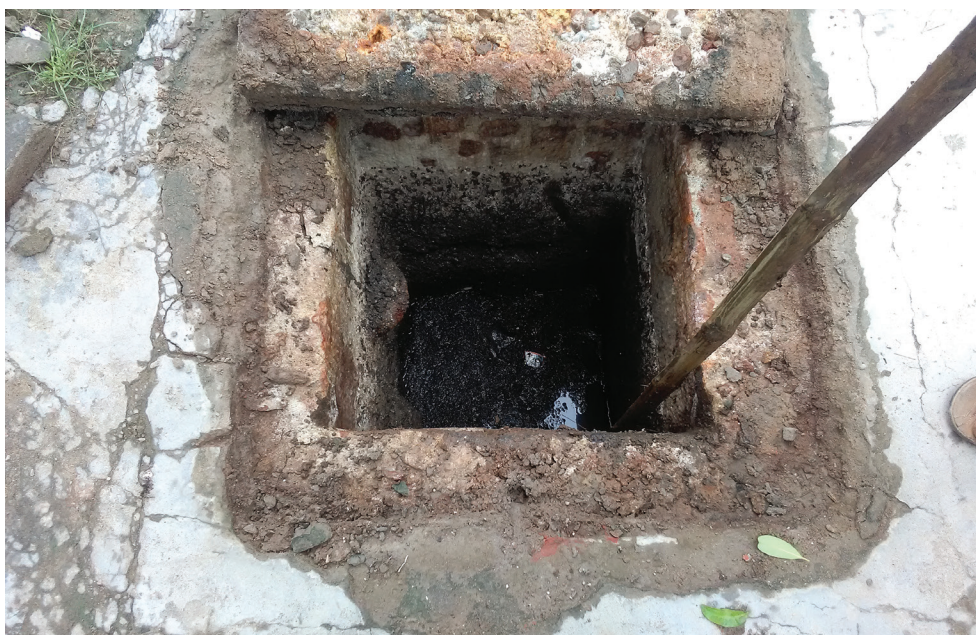
Softening of sludge through stick for emptying
