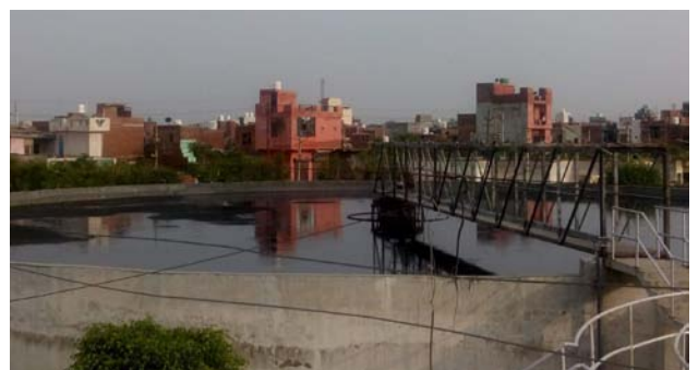
Figure 5: Sewage treatment plant working on MBBR technology
