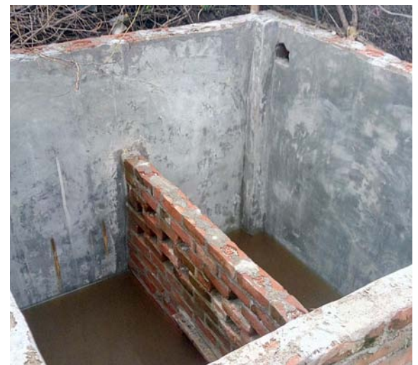
Figure 1: Septic tank connected to open drain
