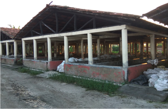
Figure 25: Sludge drying facility at FSTP (Source: Anil/CSE, 2016)
