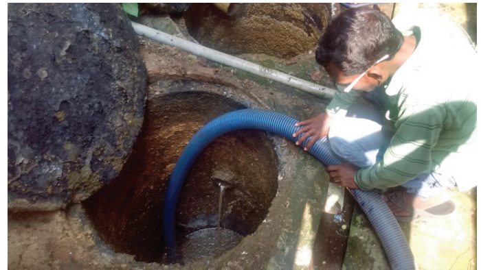
Figure 1: Emptying of a twin-pit latrine (Source: Anil/CSE, 2016)
