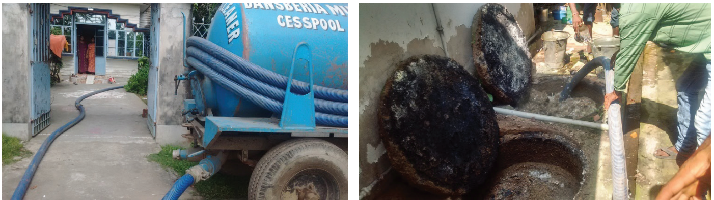
Figure 4: BM vacuum tanker used for emptying septic tank/twin pit system (Source: Anil/CSE, 2016)
