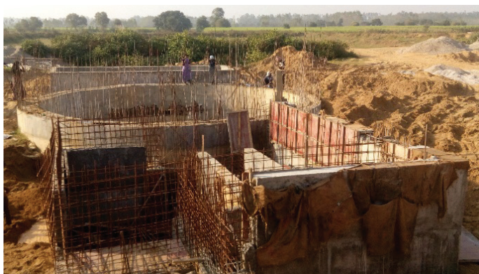
Figure 4: Screens, classifier and equalisation tank of STP under construction at Bijnor (Source: Amrita/CSE 2016)
