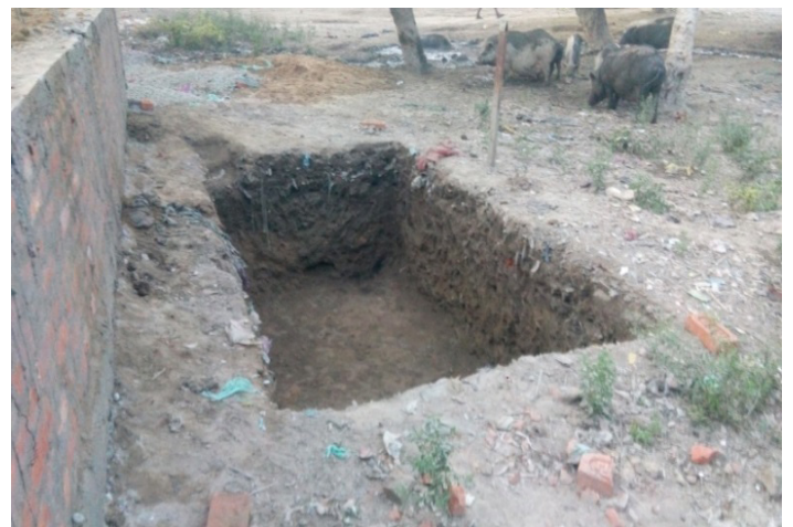
Figure 19: Containment system of community toilet at Ramrekha ghat in progress (Source: Amrita/CSE, 2016)
