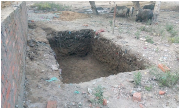
Figure 9: Septic tank of community toilet under construction at Ramrekha Ghat (Source: Amrita/CSE, 2016)
