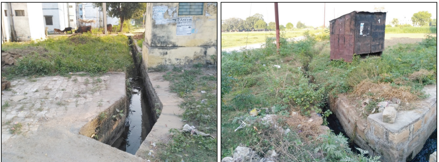
Figure 3: Wastewater conveyed through open storm-water drains (Source: Bhavik/CSE, 2016)
