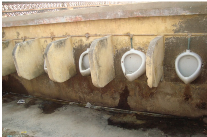
Figure 9: Men's urinals at toilet at Mishra colony (Source: Amrita/CSE, 2016)
