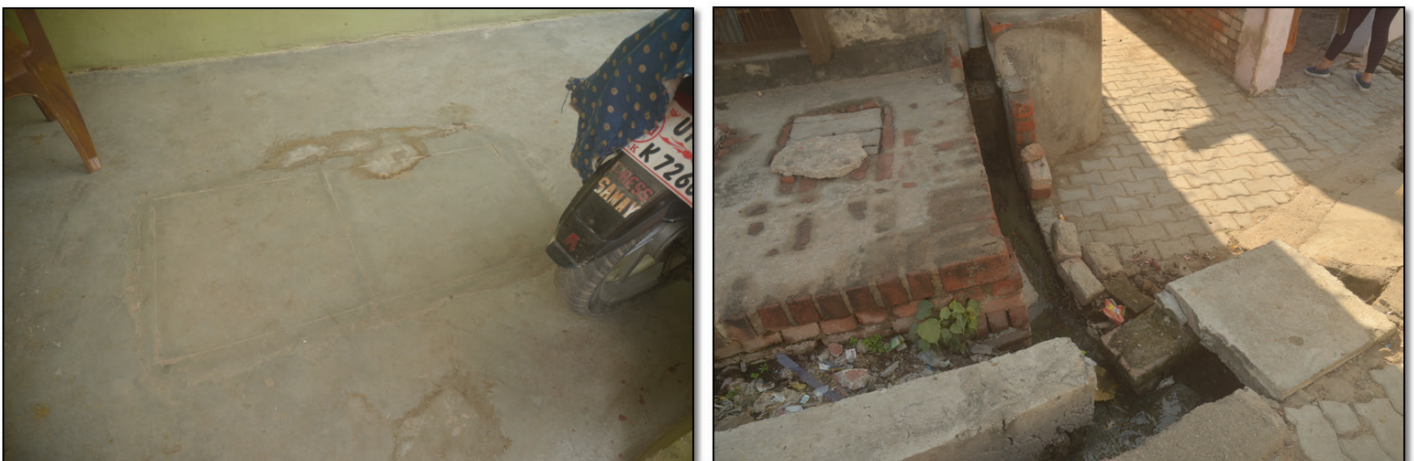
Figure 2: Containment system and its outlet (Source: Amrita/CSE, 2016)
