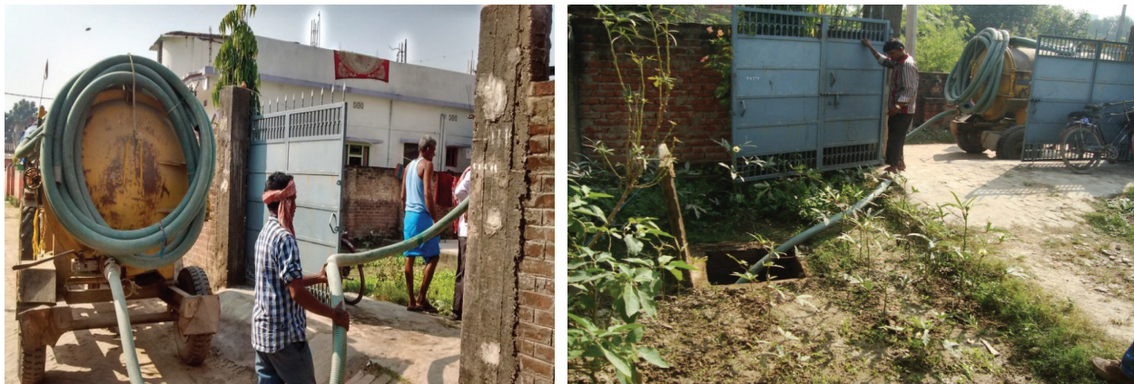
Figure 6: Emptying of soak pit containing supernatant from septic tank and grey water (Source: Anil/CSE, 2016)
