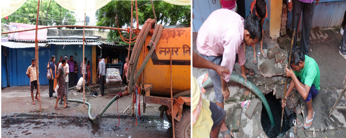
Figure 23: Emptying of clogged storm water drain (Source: Anil/CSE, 2016)
