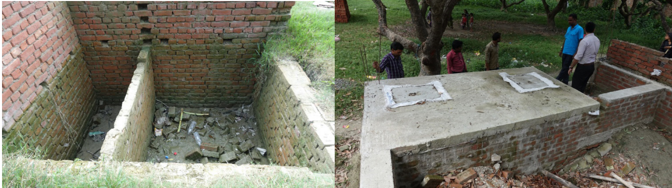
Figure 3: Septic tanks observed during field study
