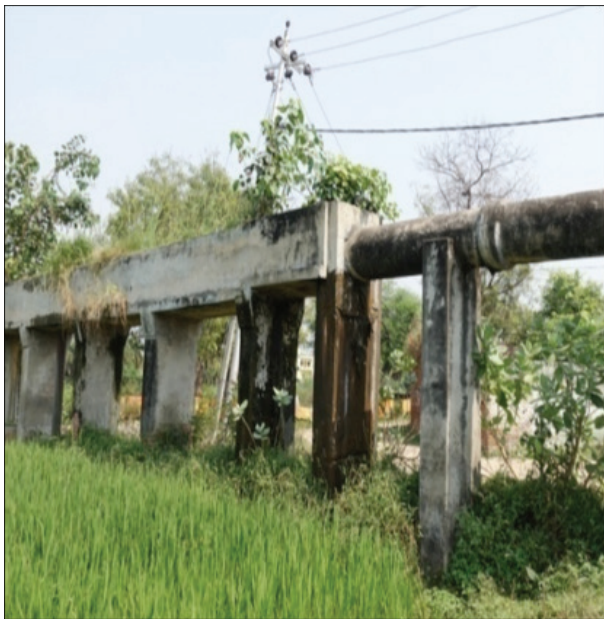
Mixing tank of sewage and tubewell water
