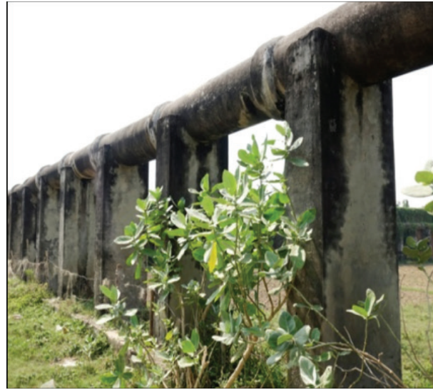
Conduit carrying sewage for irrigation
