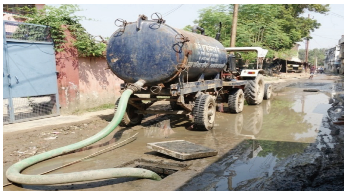
Figure 1: Vacuum tanker is used for unclogging sewers (Source: Bhavik/CSE, 2016)
