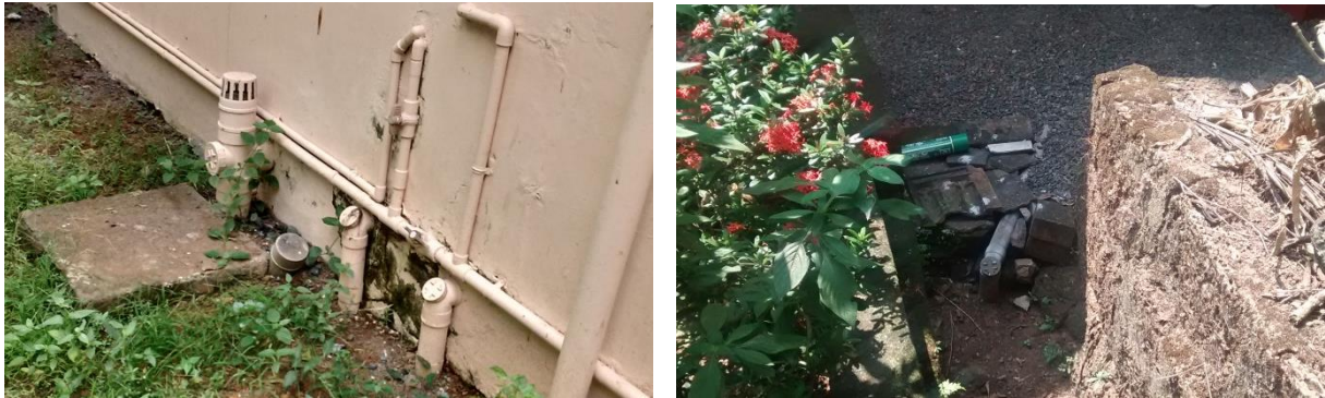
Figure 4: Grey water connected to a separately constructed soak pit (Source: Bhavik/CSE, 2016)
