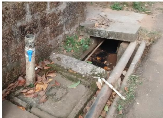
Figure 5: Grey water flowing into the open drain (Source: Anil/CSE. 2016)
