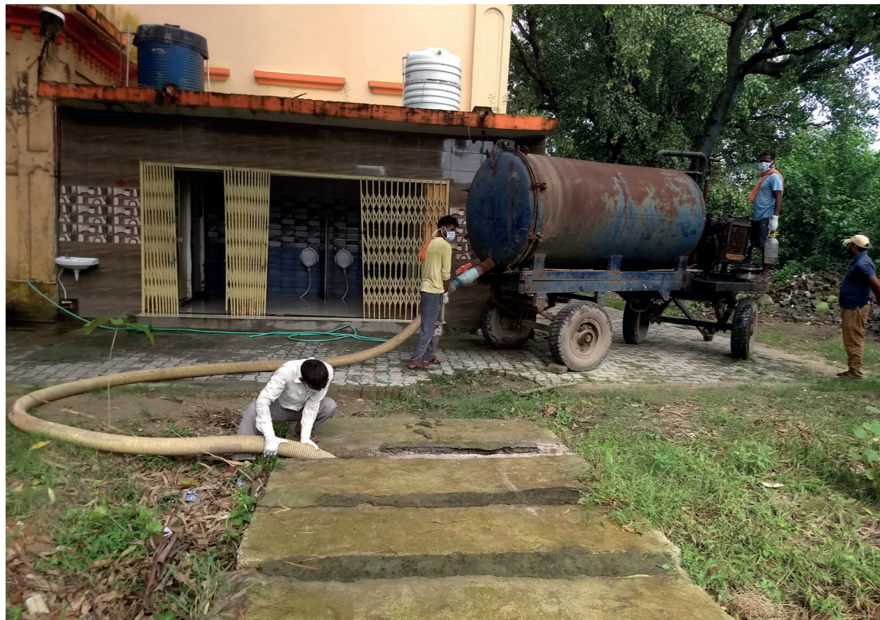
Mechanical emptying of containment system, Pilibhit
