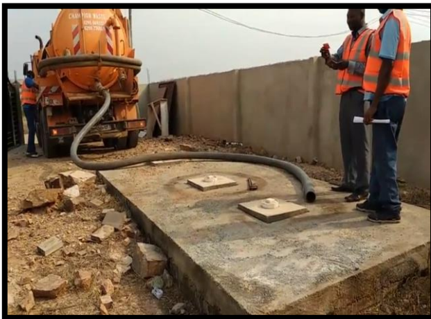
Figure 4: Septic tank with soak away at last chamber (Shantanu/CSE, 2018)
