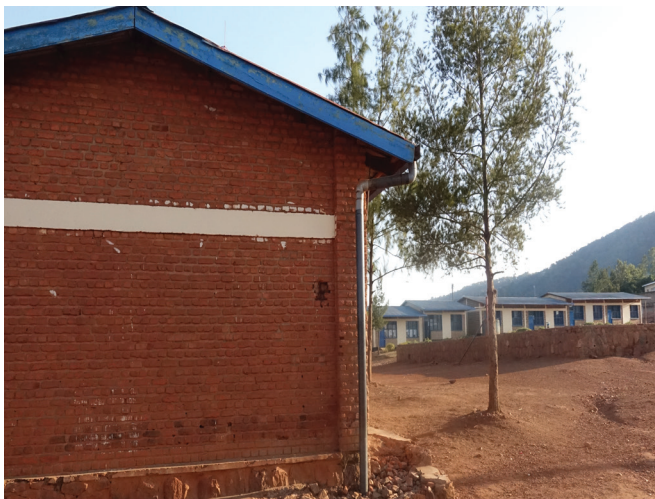
Conveyance system from rooftop to underground storage tank
