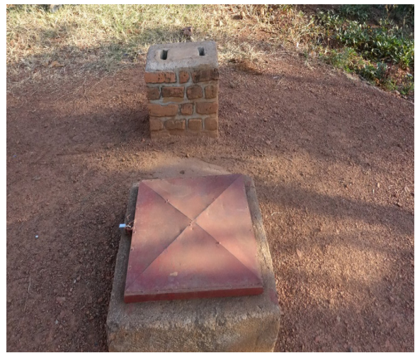
Underground storage tank
