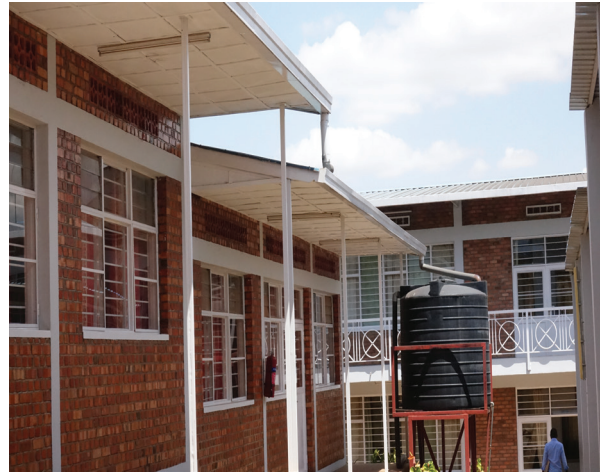
Plastic tank used for storage constructed above ground
